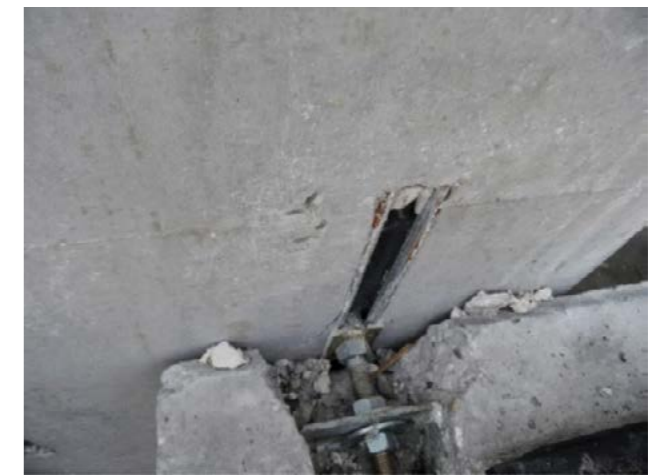
Figure 8 · Top view of the cladding-to-column connection failure [16]
