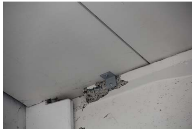
Figure 7 · Beam damage due to the roof-to-beam connection
