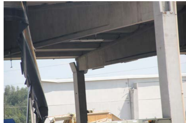
Figure 3 - Collapse of the forks at the top of the columns due to out-of-plane actions
