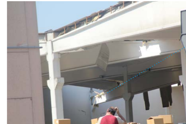
Figure 4 - Loss of support of the beam from the column
