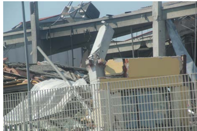
Figure 2 - Short-column effect due to the interaction with irregular masonry walls
