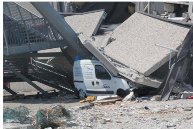
Figure 9 - Example of a collapsed cladding panel after the 2012 Emilia-Romagna Earthquake in Italy
