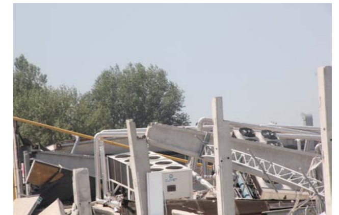
Figure 5 - Failure due to loss of support of the beam
