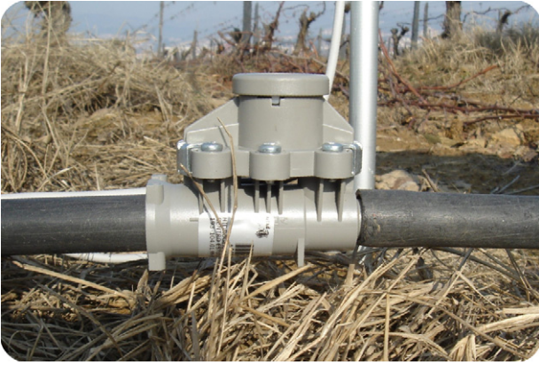
Fig. 5 – Photograph of the commercial hydrogenerator installed in a irrigation pipe.
