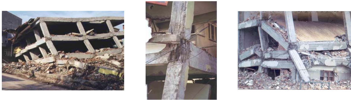
Figure 2.35 - Lack of proper design of beam-column connections (Saatcioglu et al. , 1999)
