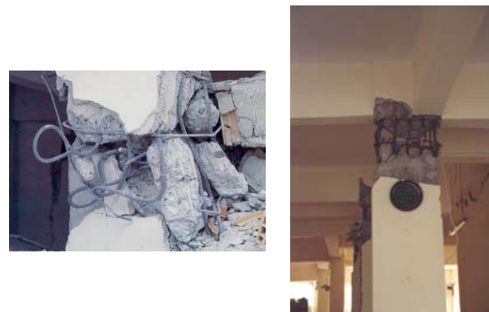
Figure 2.23 - Damaged RC columns with inadequate transverse reinforcement (Saatcioglu et al. , 1999)
