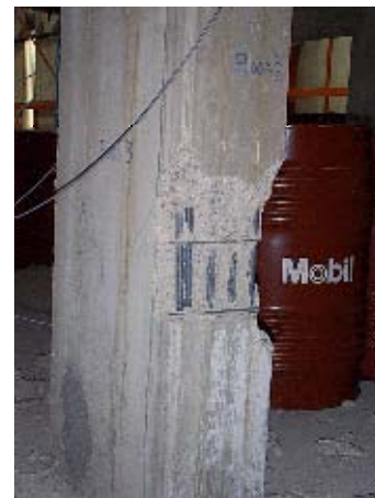
Figure B.17 - BF975: damage (spalling) at the bar termination zone of the 3 rd storey strong-column
