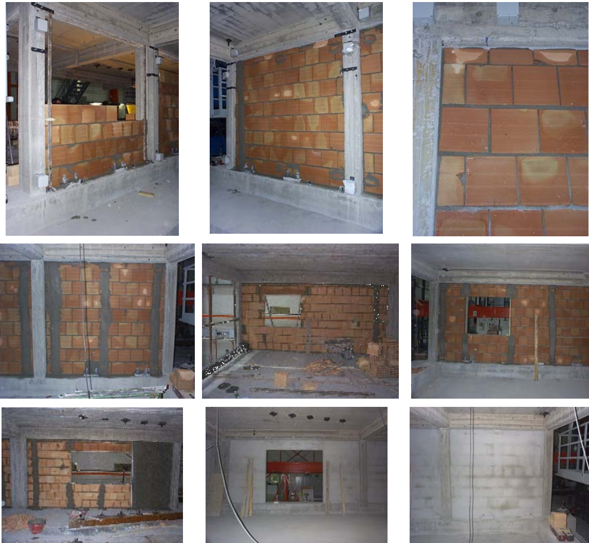
Figure A.26 - Construction of the infill masonry walls: sequential phases and detail
