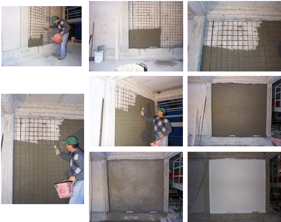
Figure A.28 - Infill strengthening construction: sequential operations and details of the reinforcing steel mesh
