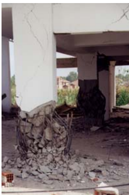
Figure 2.24 - Inadequate lap-splice and lack of stirrups (Saatcioglu et al. , 1999)
