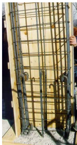
Figure 4.9 - Strong-column at the base of the 3 rd storey: lap-splice reinforcement detail (70 cm length)
