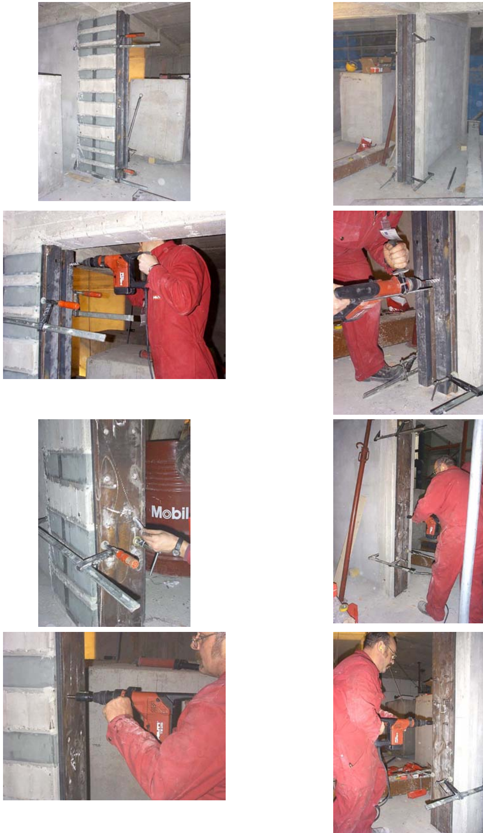
Figure A.46 - Columns drilling: strong-column (left) and weak column (right)
