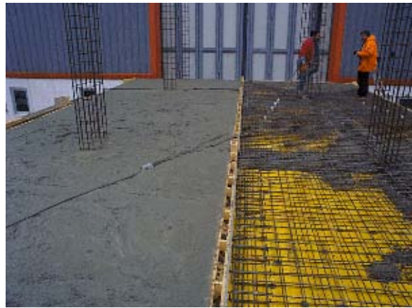
Figure A.8 - Casting of the 1 st floor (general view): the 1 st to 2 nd floor transition without lap-splice in the columns reinforcement.
