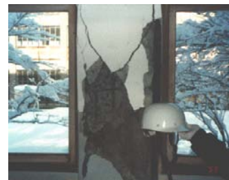
Figure 2.32 - Shear cracks at the RC column of an old school building (Yamazaki, 1993)
