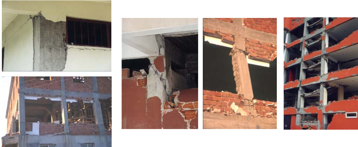
Figure 2.38 - Short column effect caused by: window opening; masonry walls; and, landing slabs of staircases (Saatcioglu et al. , 1999; Aschheim, 2001)
