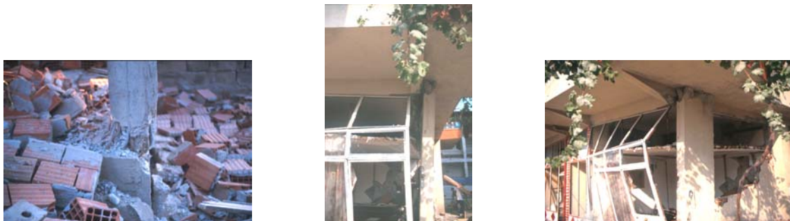
Figure 2.34 - Typical flexural failure: column hinging (Aschheim, 2001)
