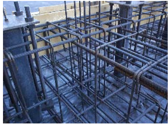
Figure A.2 - Base foundation (detail): slender-column reinforcement and tubes to apply the vertical jacks (for structure uplift)
