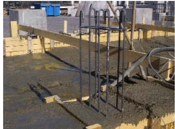
Figure A.4 - Base foundation (concrete casting) and column longitudinal reinforcement at the base with 180^\circ bends
