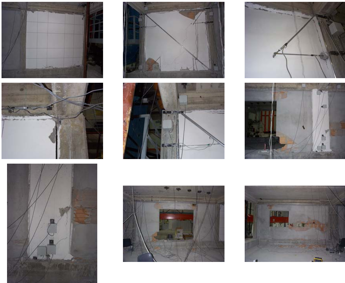
Figure B.23 - Damage on the reinforced concrete frame, infill and infill strengthened panels after the SC earthquake tests
