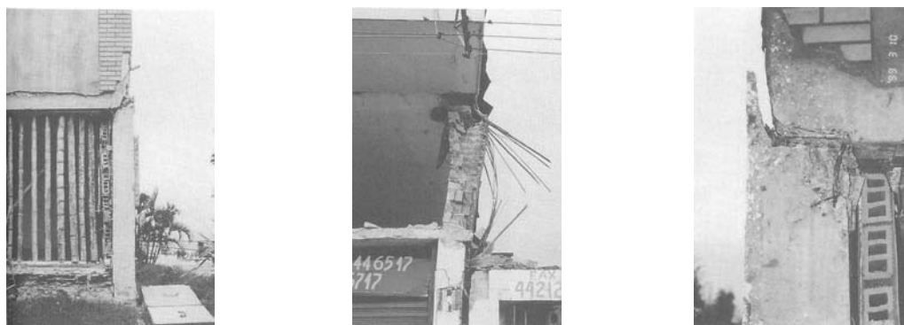
Figure 2.16 - Poor reinforcing details in RC joints (Kagami, 1999)
