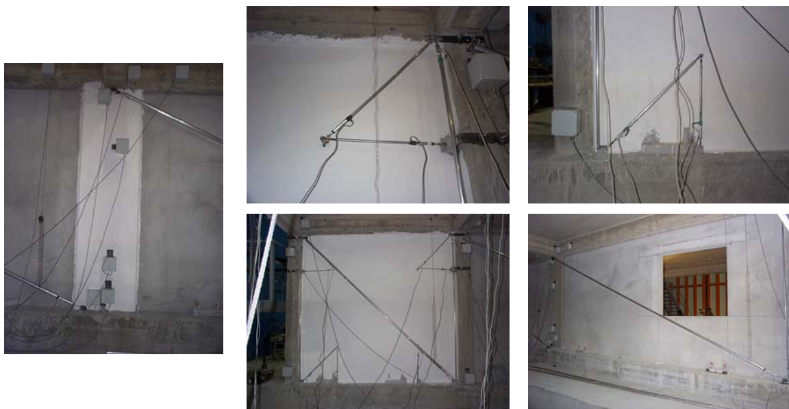
Figure A.29 - Infills instrumentation installed for the IN and SC tests: panels and local instrumentation at the panel corners of the short external panel
