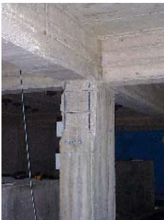
Figure B.16 - BF975: damage (spalling) at the top of the 3 rd storey strong-column
