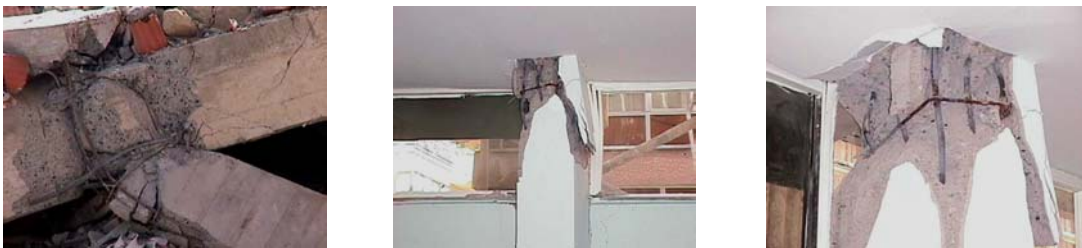
Figure 2.12 - Damage in buildings due to inappropriate detailing (KOERI, 1999)
