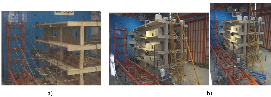
Figure A.27 - Four-storey full-scale reinforced concrete infilled frame: a) construction of the masonry infill walls; b) general views of the structure
