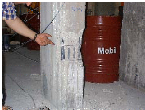
Figure B.15 - BF975: damage (spalling) at the bar termination zone of the 3 rd storey strong-column
