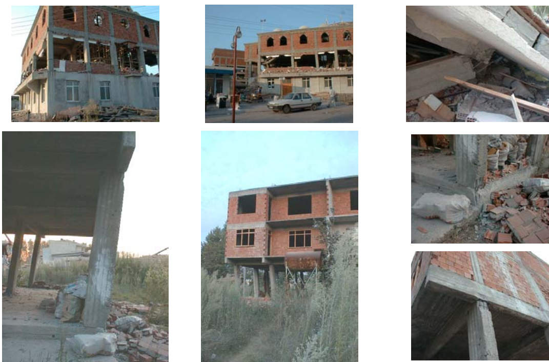
Figure 2.13 - Damage in RC buildings under construction after the Izmit earthquake (EQE, 1999)
