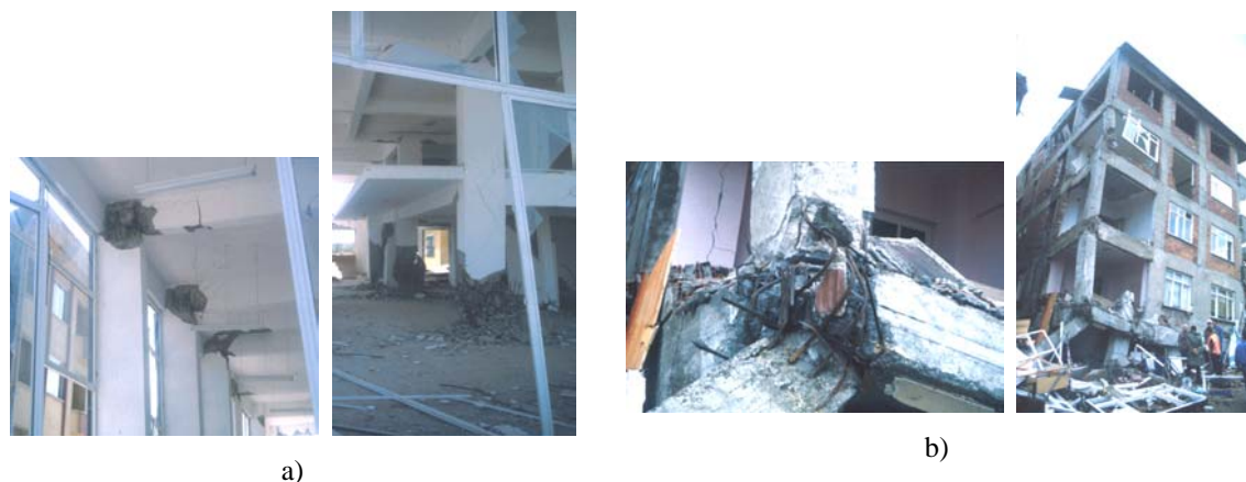
Figure 2.36 - Inadequate strength of joints (Aschheim, 2001): a) joint damages; b) joint failures
