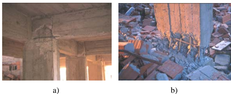
Figure 2.25 - Typical deficiencies in buildings: a) beam bars terminate with tight 180° hooks in the joint; b) yielding of the longitudinal steel adjacent to the floor slab (Aschheim, 2001)
