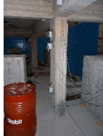
Figure B.14 - BF975: Damage (spalling) at the top of the 3 rd storey strong-column (beginning)
