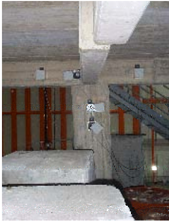
Figure B.13 - BF975: the horizontal storey displacement is evidenced (comparing the relative position of the transversal beams of the two frames)
