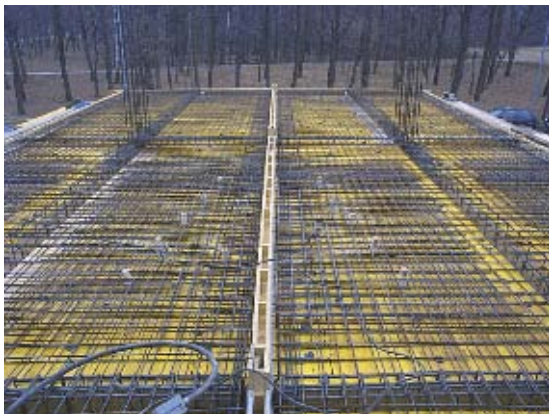
Figure A.5 - Slab reinforcement, reinforcement added in the attachment zone and plastic tubes for connection to the steel loading frame
