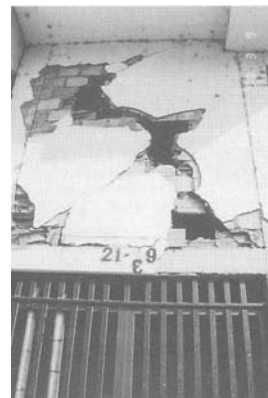
Figure 2.15 - Damage in an ordinary RC moment-resistant infilled RC frame (Kagami, 1999)
