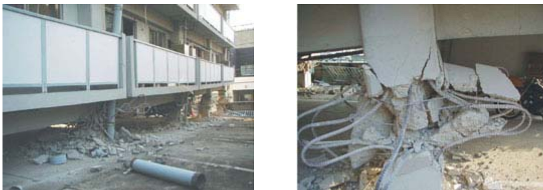
Figure 2.7 - Partial collapse of a three-storey residential building in Imabari (EQE, 2001)
