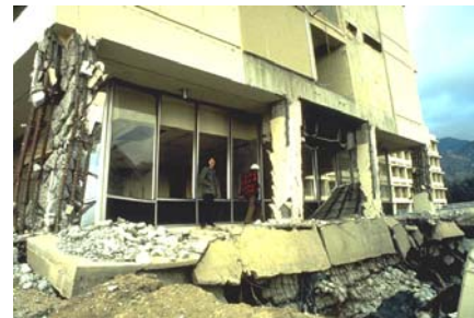
Figure 2.30 - Damaged RC corner column at the 1 st storey (Bertero, 1997)
